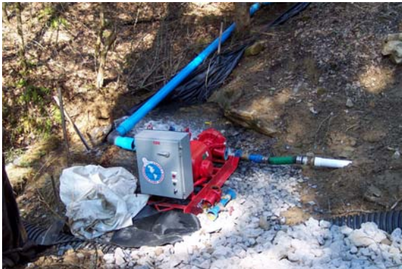
Water Supply Pump from Dam Blue Pipe is line to tanks
