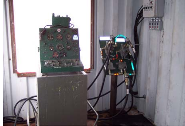
Control Stations in purpose built container
