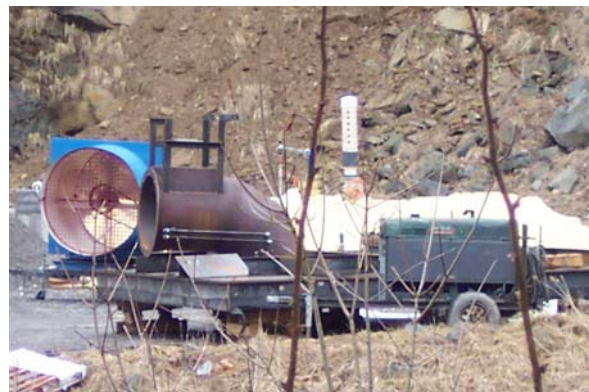
No. 7 Shaft with pressure relief fitted
